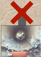
Damaged sewer pipe by dialysis drainage
